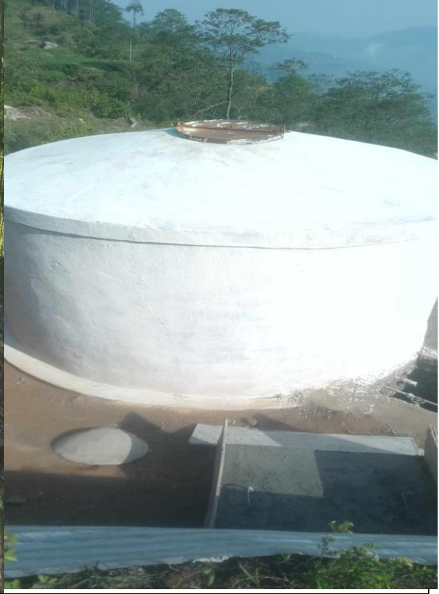
RVT Tank 14m 3
